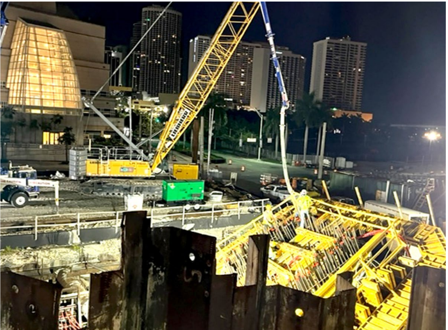
Concrete pour for a starter arch at one of the I-395 signature bridge arches
