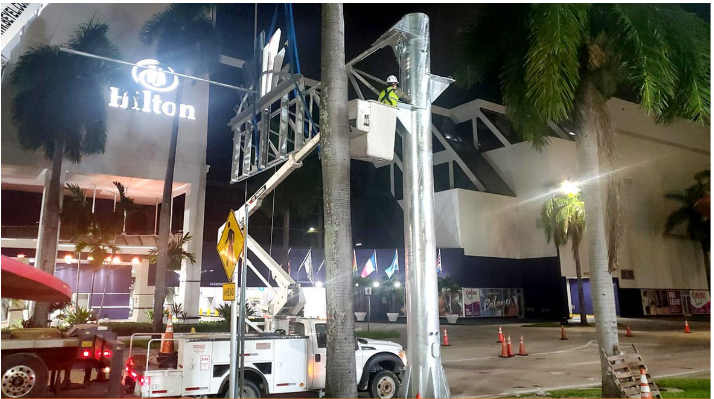
Installation of support structure for an electronic message board over Biscayne Boulevard and NE 17 Street
