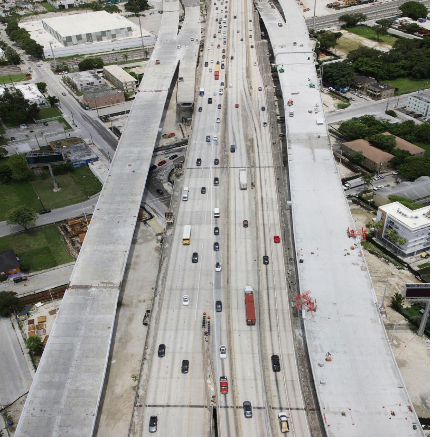
New eastbound and westbound I-395 bridges under construction just east of NW 3 Avenue
