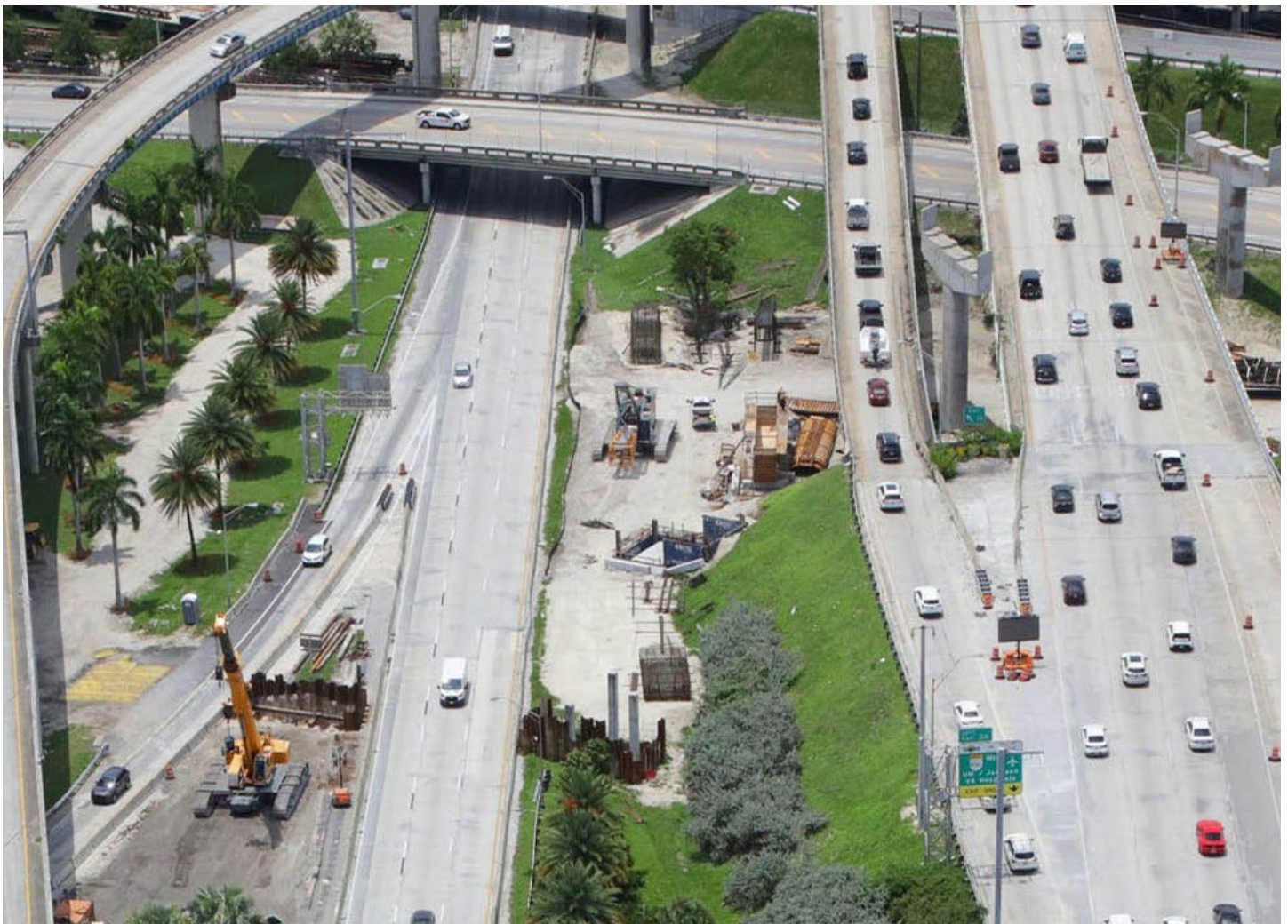
Foundation work adjacent to I-95 for the new westbound I-395 ramp to southbound I-95
