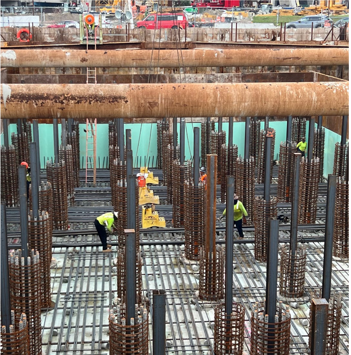
Installation of reinforcing steel at one of the signature bridge arch foundations
