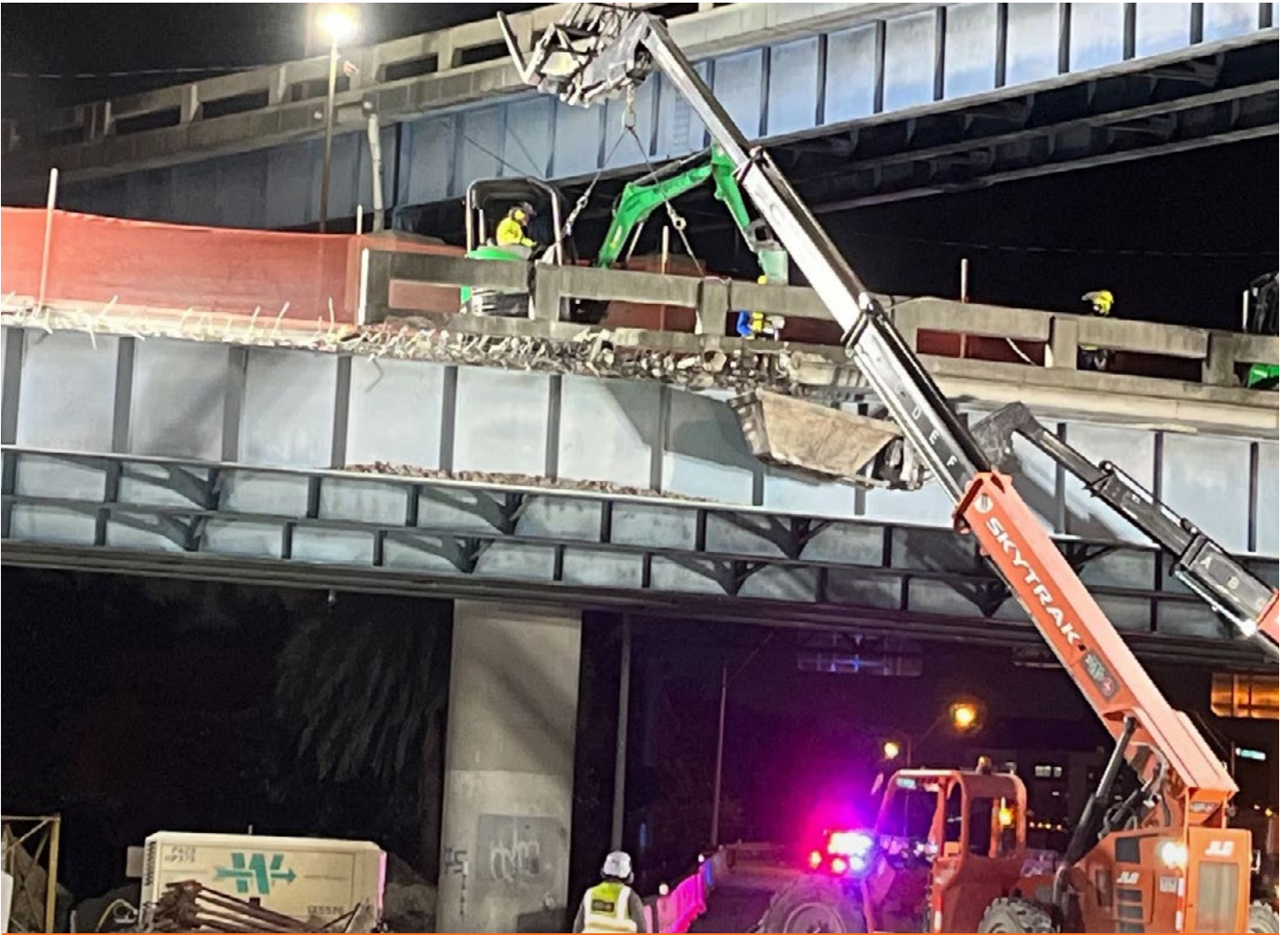
Ongoing work to replace traffic railing on the eastbound SR 836 ramp to northbound I-95
