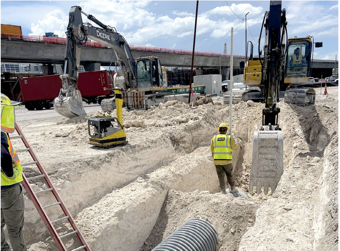
Ongoing drainage work on NE 13 Street between NE 2 Avenue and NE 1 Avenue
