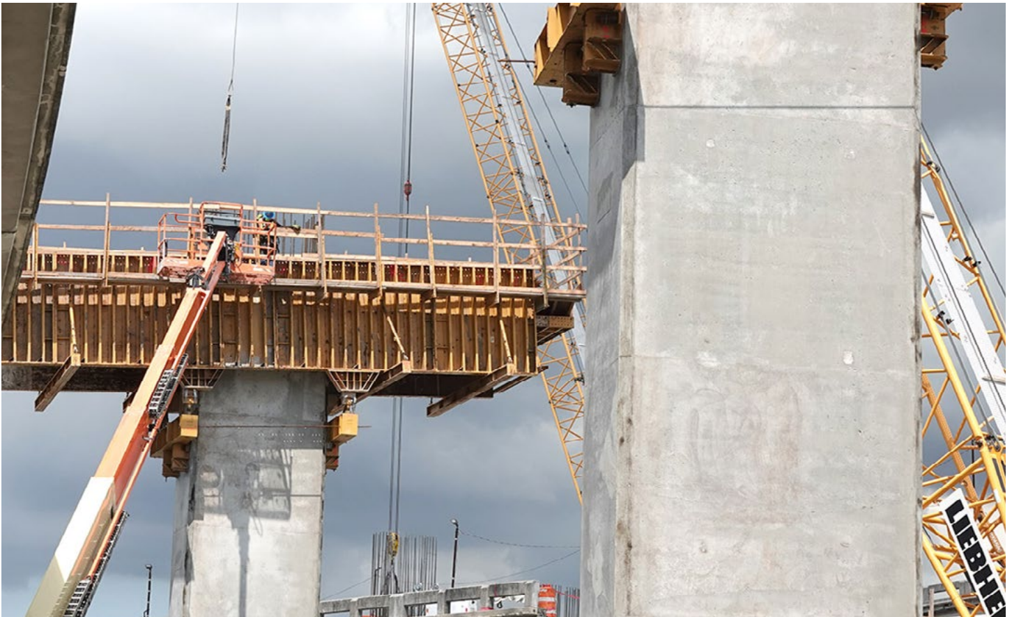
Pier cap construction for the new SR 836 double decked roadway at the core of the interchange
