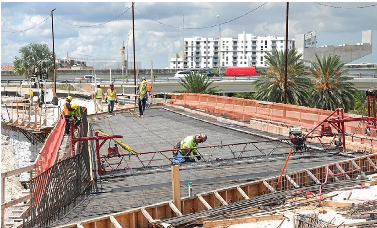
Ongoing work to prepare the new northbound I-95 ramp to eastbound I-395 for the concrete deck pour
