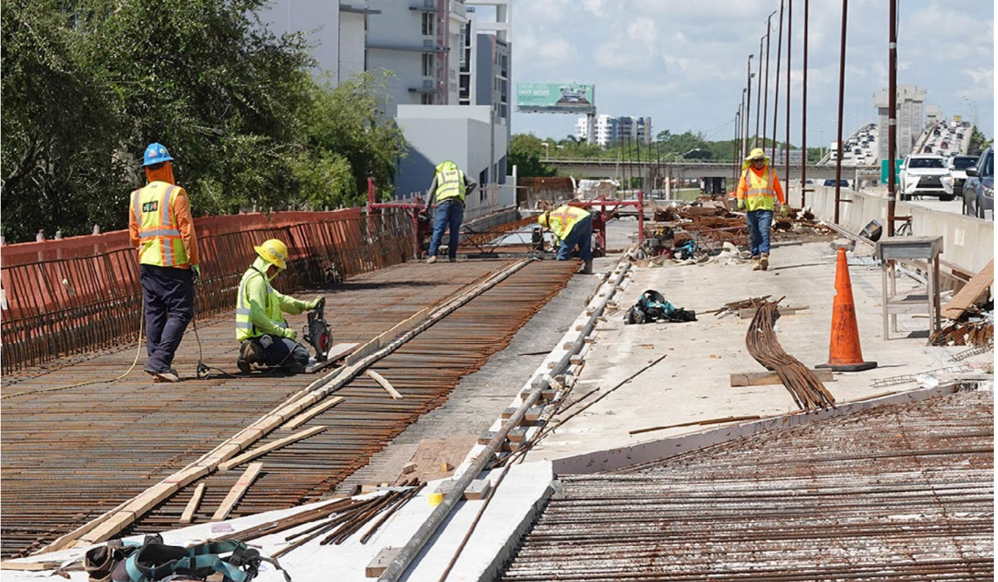
Preparation of roadway deck for concrete placement on eastbound SR 836 just west of I-95
