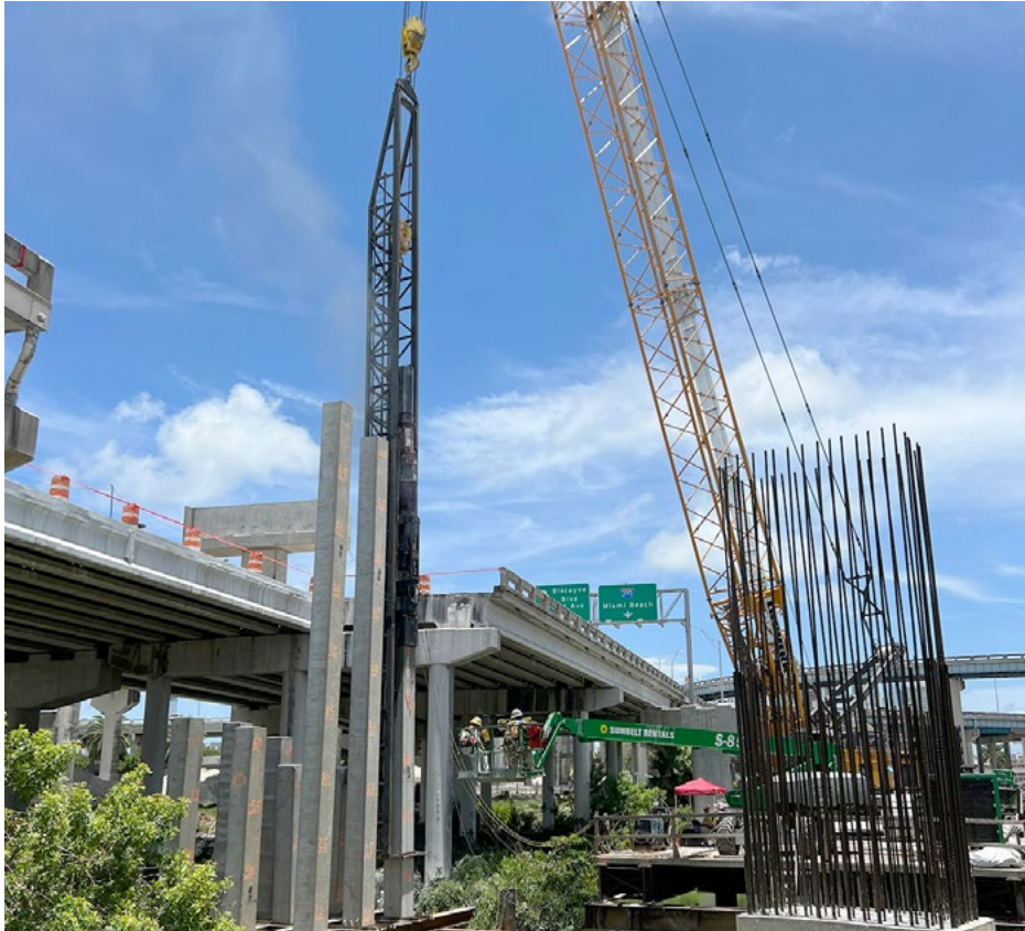
Crews driving concrete piles into the ground for an SR 836 double decked bridge foundation.
