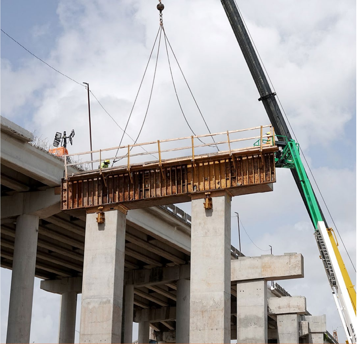
Construction of I-395 pier cap for a temporary bridge to connect I-395 with SR 836 and southbound I-95
