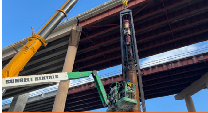
Driving pipe piles in the Miami River for the construction of a temporary trestle bridge
