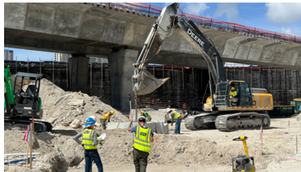
Crews installing drainage structures at future approach to the westbound I-395 entrance ramp at North Miami Avenue
