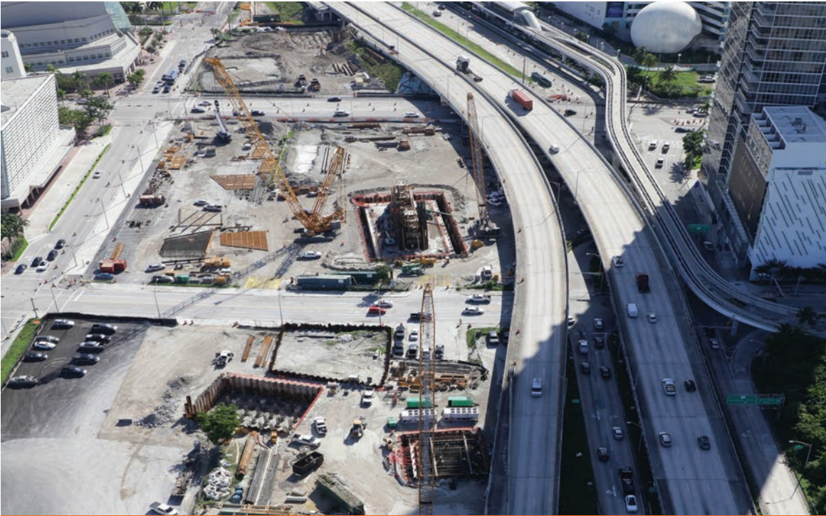
Aerial photo showing the Signature Bridge center pier footer and four bridge arch footers
